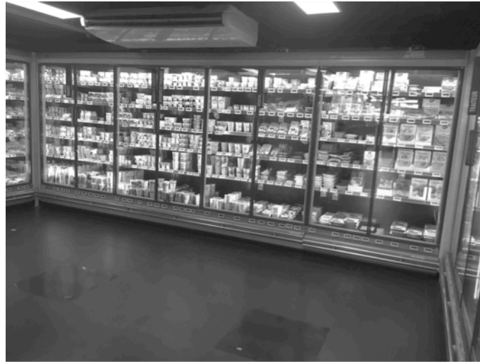
Figure 3: Soundwalk at Place Castellane, March 24, 2021. Listening to the device of the organic store: refrigerators arranged in a "U", neon lights and air conditioning (photo by Caroline Boë)
